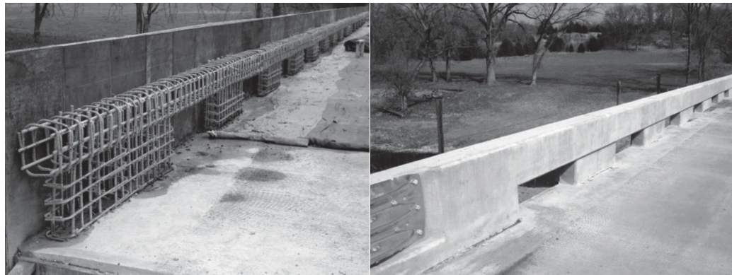
Figure 3.4 - Reconstruction of Bridge No. 14802301 (a) GFRP reinforcement cages prior to casting of railing, (b) open-post railing in service.
